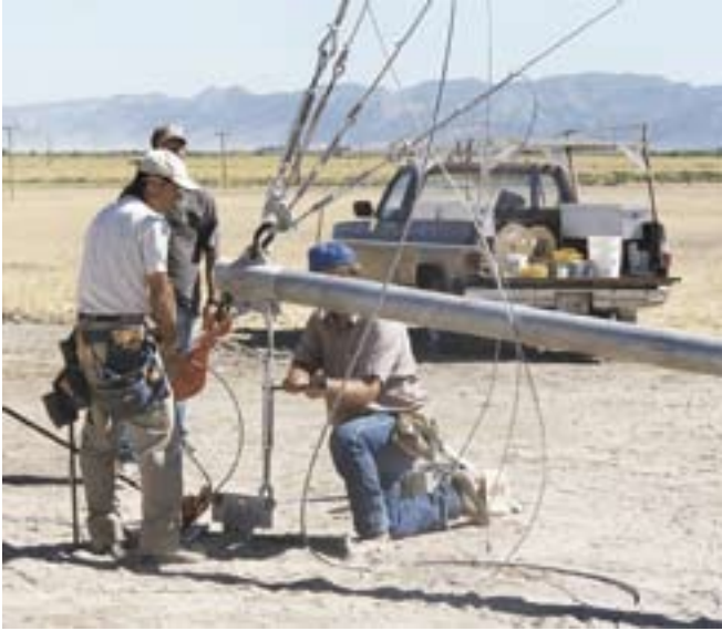
Gin pole down, tower up—with careful measuring, the gin pole turnbuckle will come out plumb, making tensioning easier.
